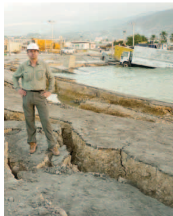
Marc Eberhard stands on collapsed pavement.
